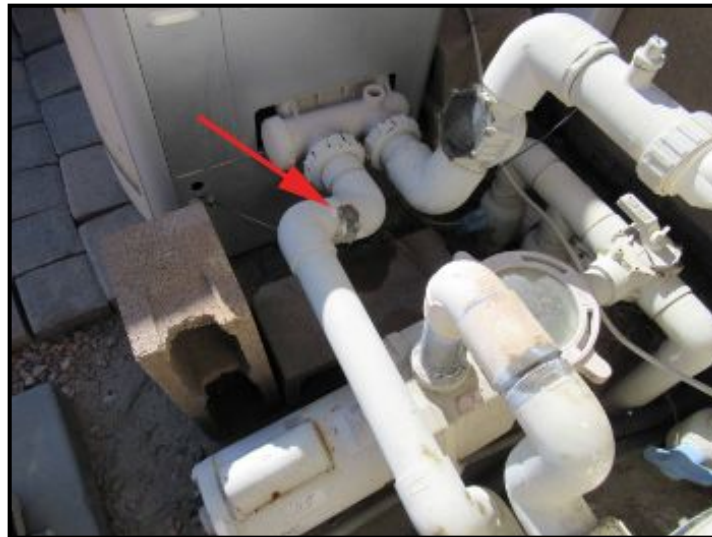
Leak in heater inlet line - recommend repair
