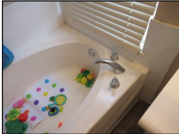
Leaky faucet in master bath - recommend repair.
