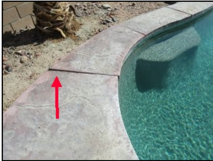
Section of concrete slightly lifted by old palm tree
